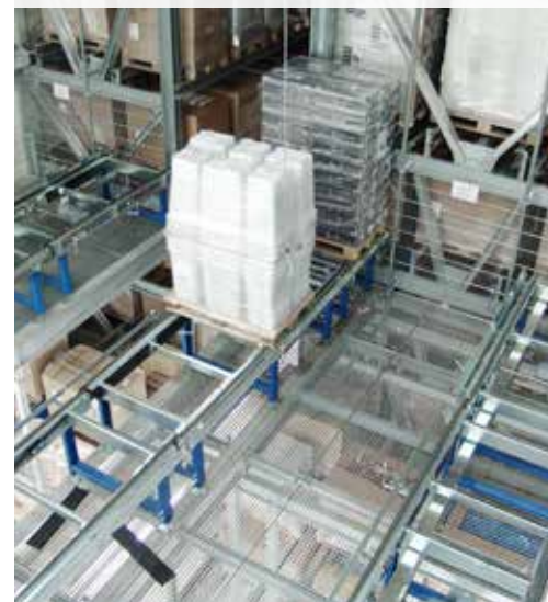
High-bay warehouse with 11,600 pallet storage locations
