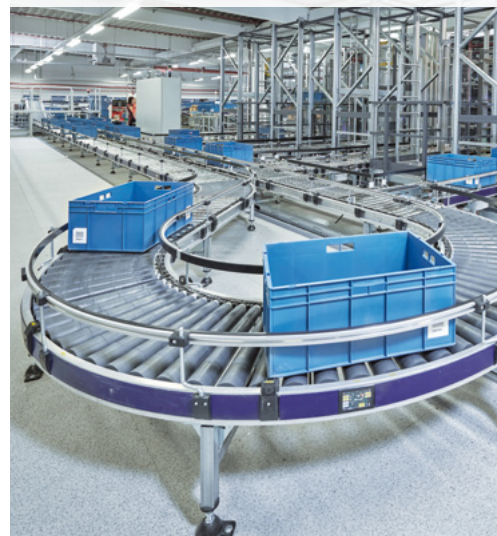
Pre-zone of the shuttle storage system
