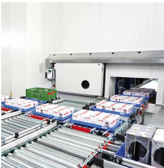
Airlock with conveyor technology
