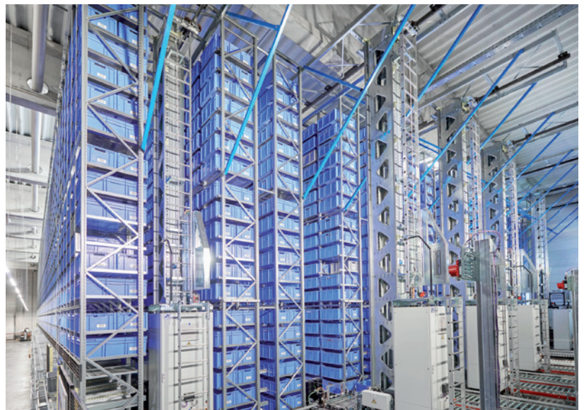
7-aisle, automated small-parts warehouse with 31,920 bin storage locations
